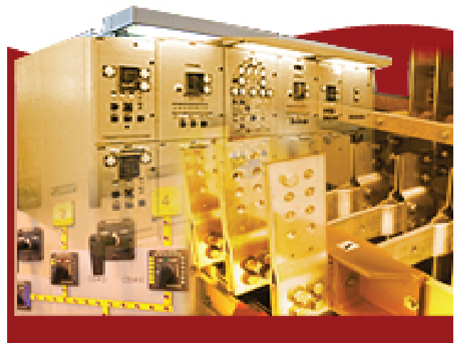
Two sets of one-piece, two-section low-voltage distribution switchgear were installed.
