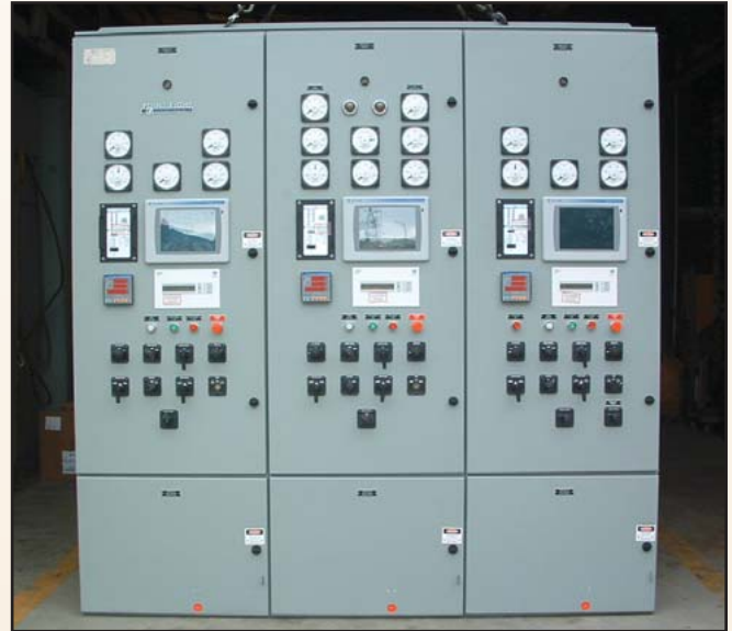
A 480-V UL 891 generator control switchgear on Ship Shoal 332B.
