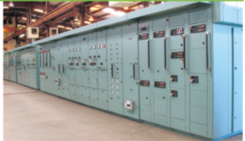
▲ Pictured above are low voltage distribution boards close coupled to motor control centers built to American Bureau of Shipping standards.
