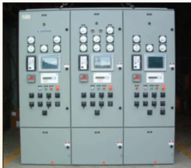
A 480-V UL 891 generator control switchgear on Ship Shoal 332B.
